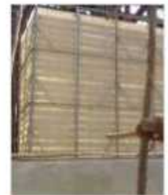
NATURAL DRAFT COOLING TOWERS
