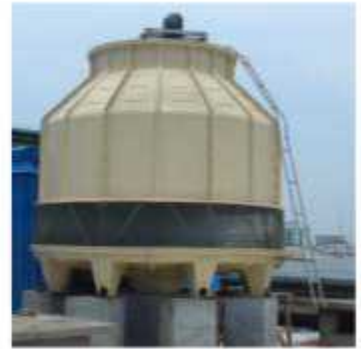
150 TR HVAC APPLICATION - COLOMBO (2012)
