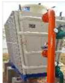
DRY COOLING TOWERS
