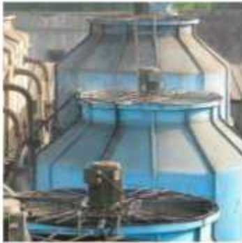
400 TR - 5 Nos STEEL MELTING PLANT - CHENNAI (2010)
