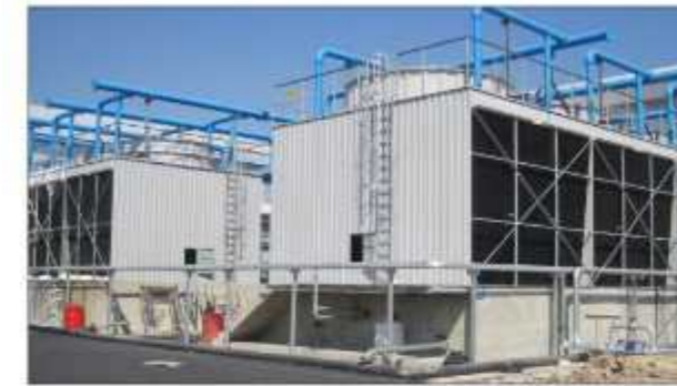
DFT-1500 m 3 / hr x 2 OIL REFINERY DAMMAM
