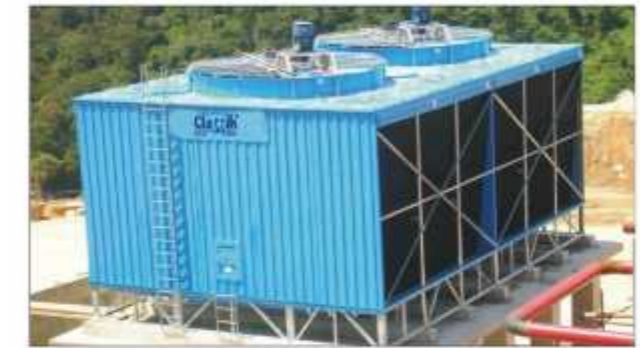
DFT-700 m 3 / hr x 2 CENTRAL PROJECT MALAYSIA
