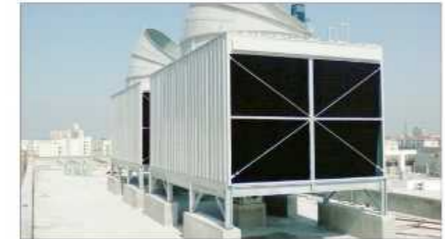
DFT-500 m 3 / hr x 2 WATER PROJECT RIYADH
