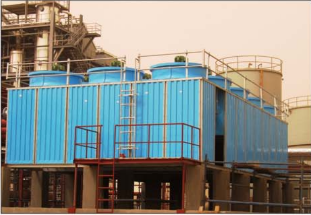
Oil Refinery - Saudi Arabia - 3600 TR
