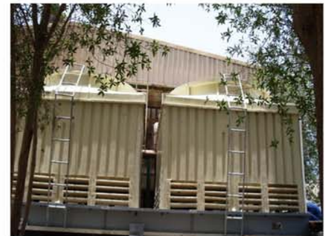
Towers at Site
